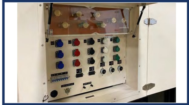
CUSTOMER CONNECTION PANEL
